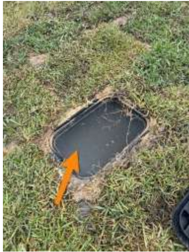
Standing water in valve
